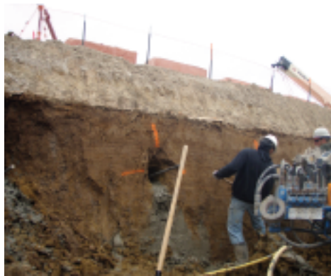
Figure 6. Photograph illustrating the sloughing of soil during the first lift drilling of the soil nails
